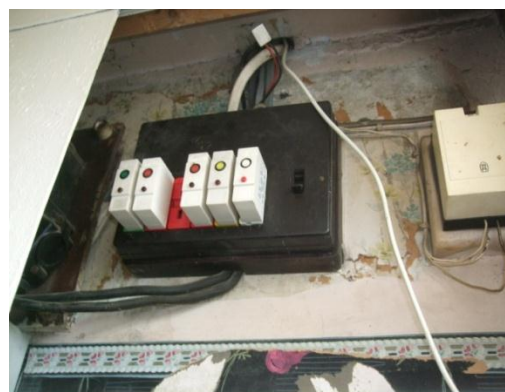
Fuse board, dated and no earthing
