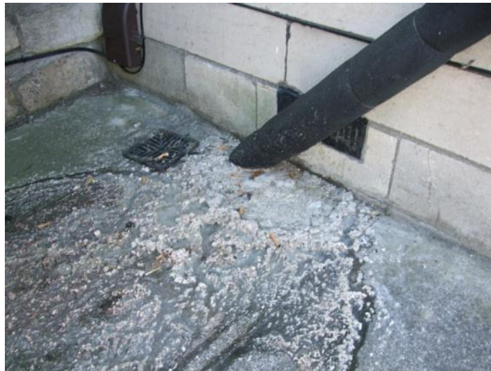
Blocked front drain
