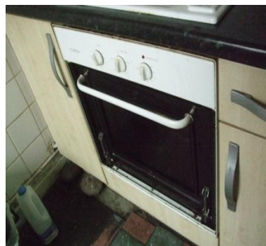
Front panel missing off oven
