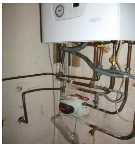
Unsafe boiler potentially leading to carbon monoxide poisoning and explosion
