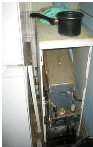
Damaged boiler with front panel missing
