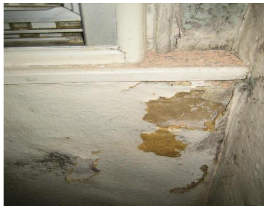
Damp leading to mould and potentially mental and social health effects
