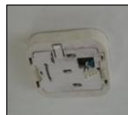
Disabled smoke alarm with the cover removed
